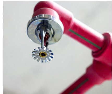
Fire Sprinklers System
