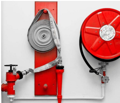
Fire Hose Reel & Breaching Inlet System
