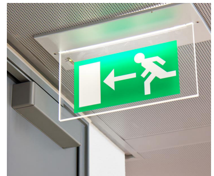
Emergency & Exit Lights System
