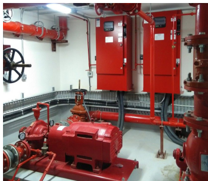
Fire Pump System
